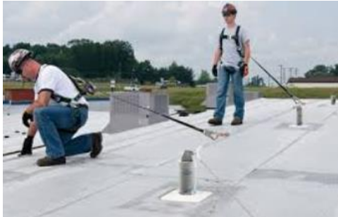
Figure 57 – Fixed static line on roof
